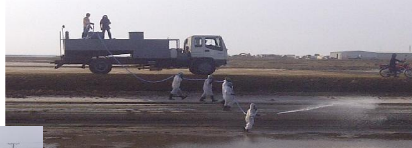
Disinfection of wet areas
