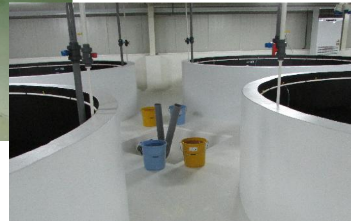
Individual tank equipment
